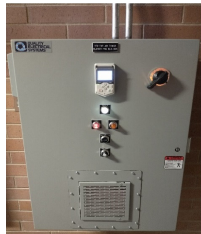
New VFD for air blower
