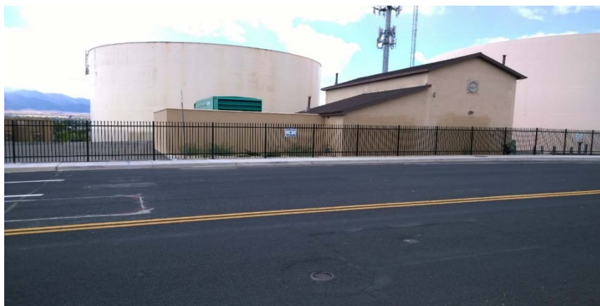
New generator, sound wall, sidewalk & fence
