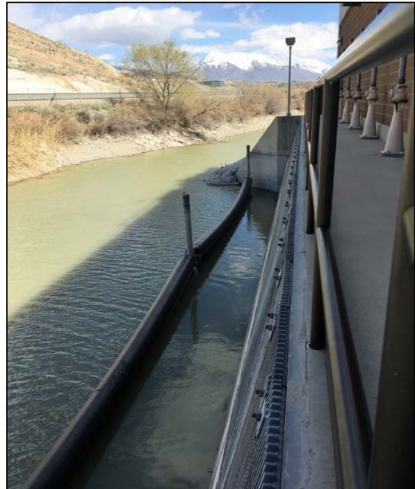
New JNPS floating debris screen
