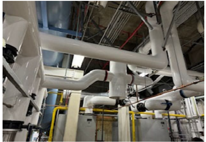
New Boilers Piping
