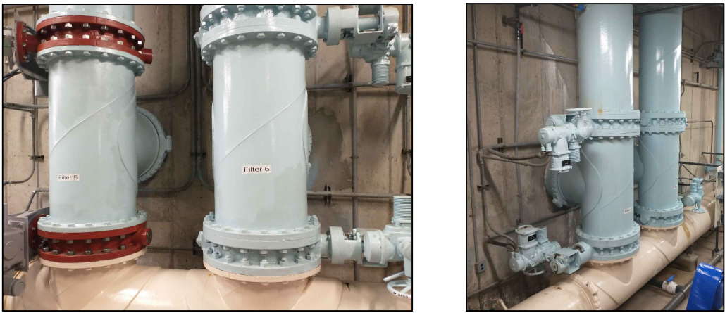
EXISTING VALVES AND ACTUATORS
