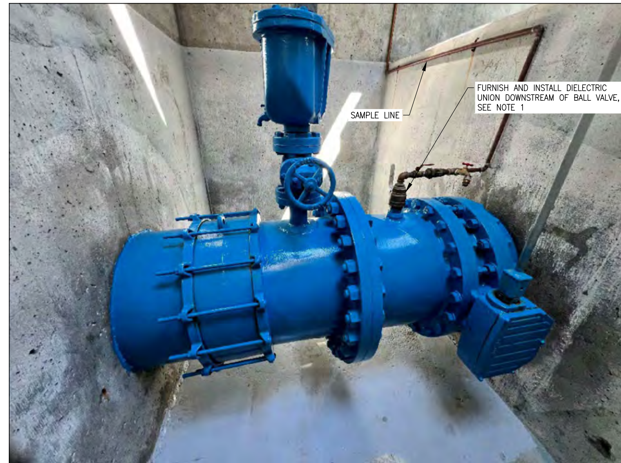
IMAGE OF JA-2 11400 SOUTH TURNOUT VAULT NTS
