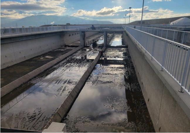
Sedimentation basin with old sludge collection equipment removed
