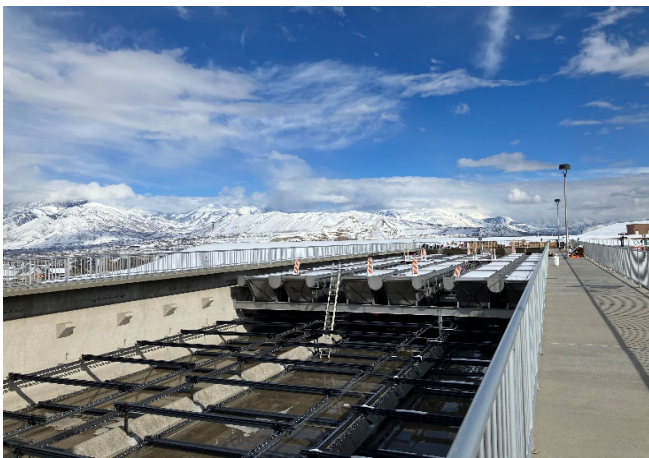
Installed sludge collection equipment and plate packs
