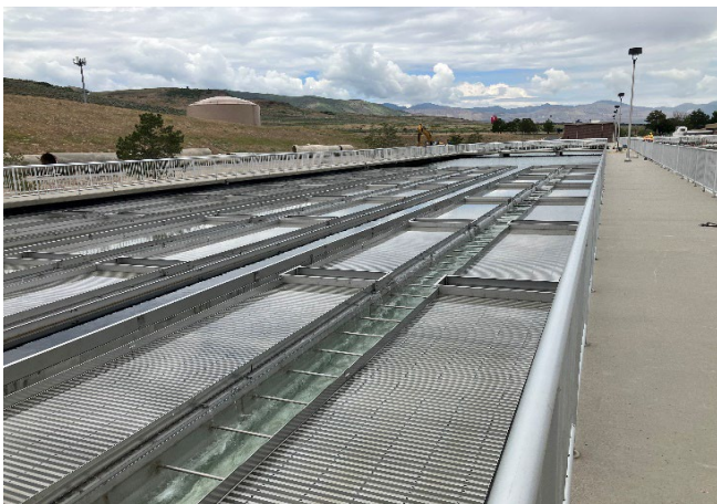
Operating plate settlers
