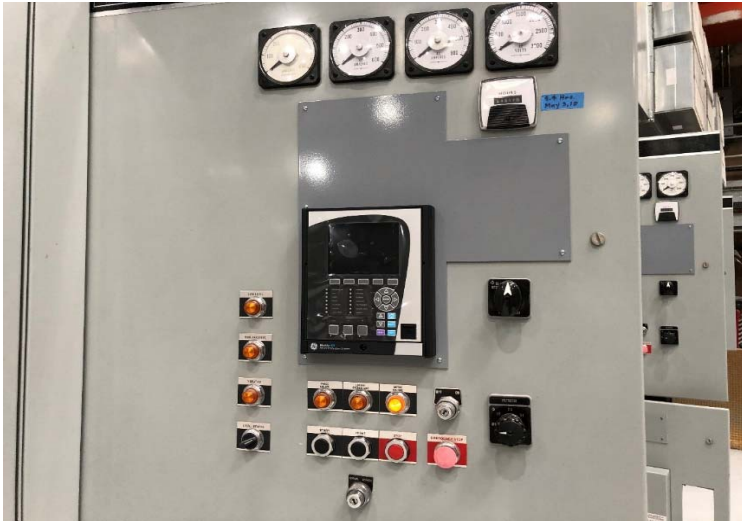
New pump control panels for remote operation.
