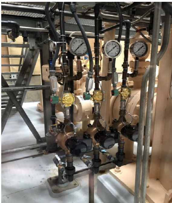
Pump monitoring equipment which is connected to SCADA for remote control.
