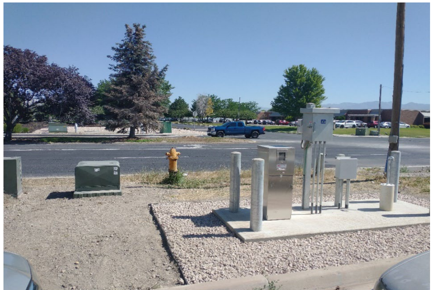
Finished construction with new transformer, pad, power meter, rectifier, and cathodic well.
