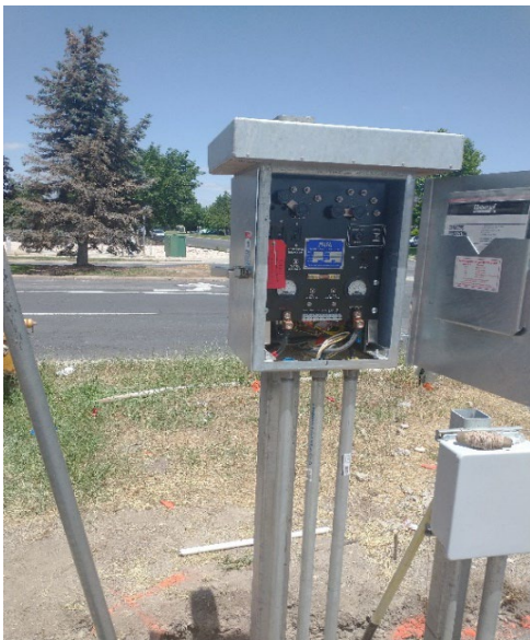
New cathodic rectifier
