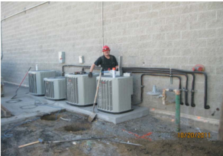
New Condensing Units.
