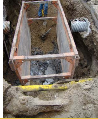
Contaminated soils near 5600 South 900 East
