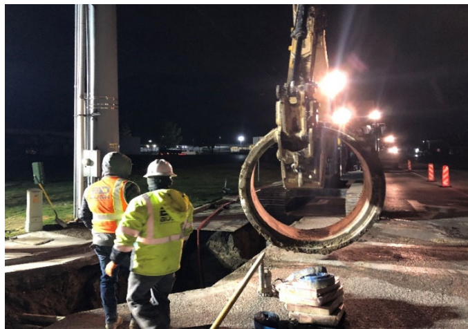
Abandonment of a valve vault from 1956
