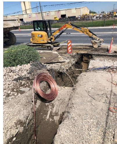
New 3/4" service lateral
