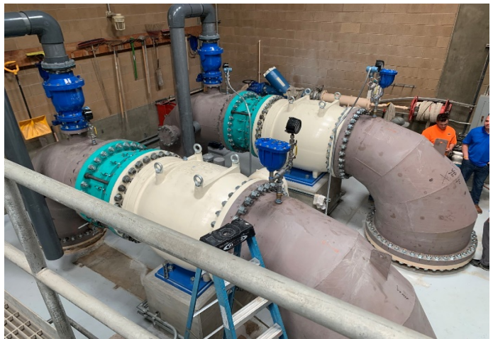
JNPS flow control valves
