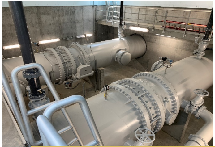
JVWTP SWA-1 connection vault
