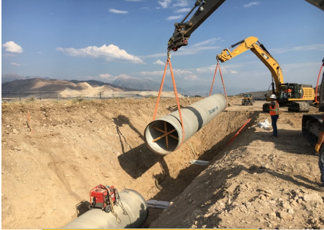
Installation of 66" mainline steel pipe located between Redwood Road and Porter Rockwell Boulevard
