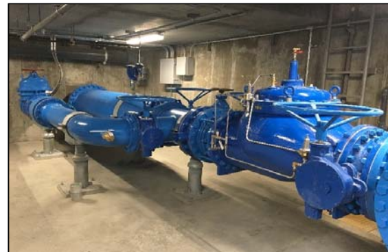
Completed Vault Piping
