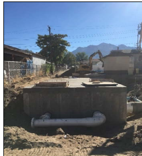
Flow Control & Meter Station Vault
