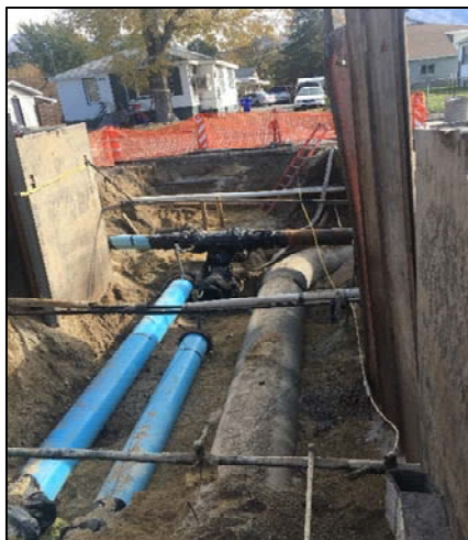
16-inch, 14-inch, & 30-inch Pipelines
