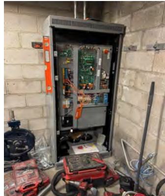
New Elevator Control
