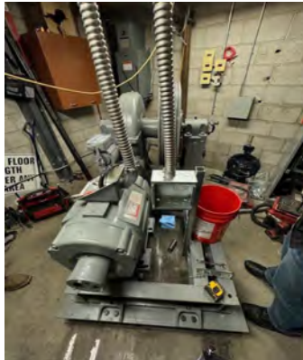
New Elevator Motor
