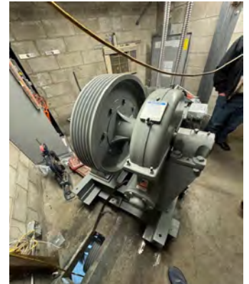
New Elevator Gear
