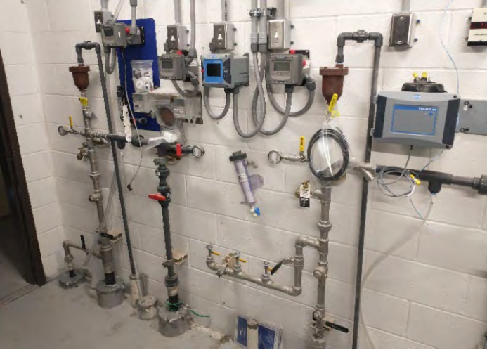
Monitoring Equipment in new Chemical Building
