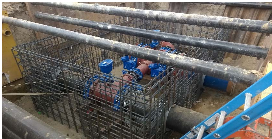
New valve vault at 3785 West
