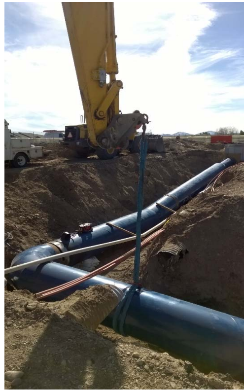
New 36-inch steel pipe at pump station
