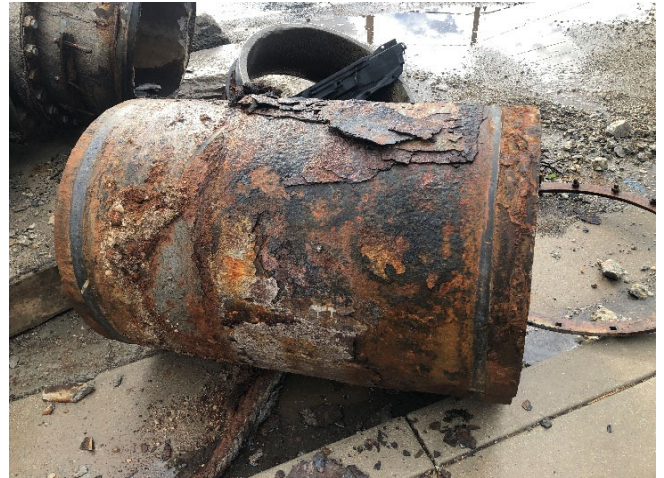
Corroded section of existing 30" piping
