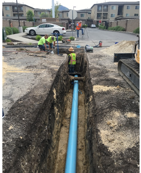
Fire line connection on 200 East.
