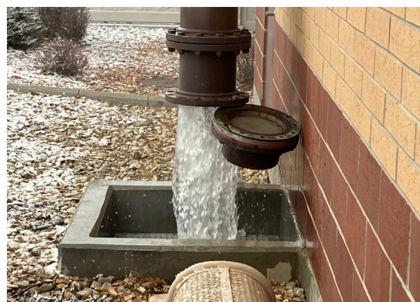
DW7 producing clear water
