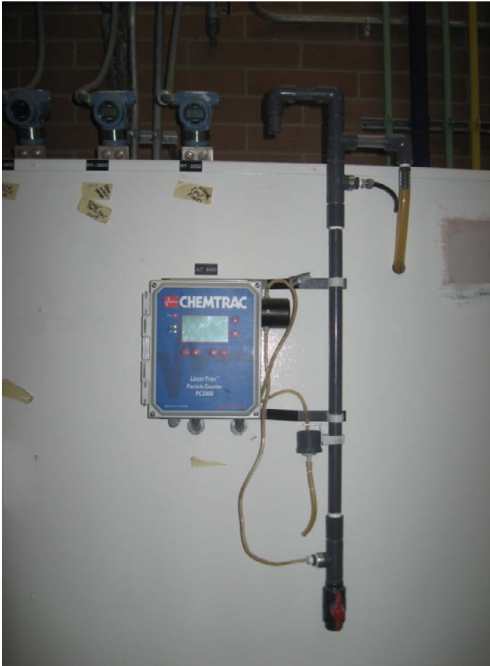
Chemtrac Particle Counter Unit - SWGWTP
