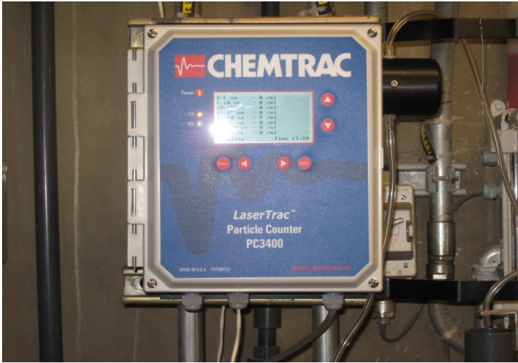
Chemtrac Particle Counter Unit - SERWTP
