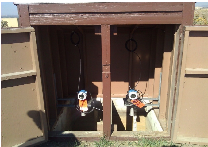
New Water Level Sensors
