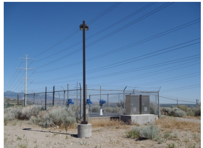
Actuators, RTU Cabinets, and New Light
