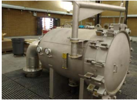
RO Pretreatment Equipment
