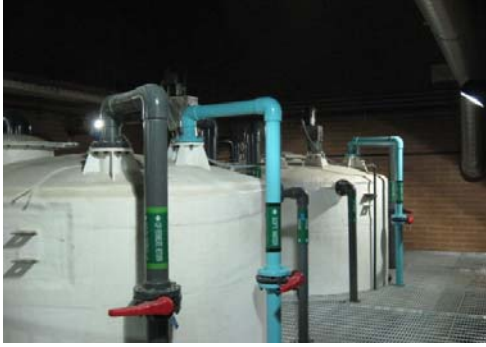
Clean in Place System
