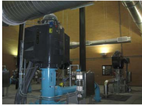
RO Feed Pumps
