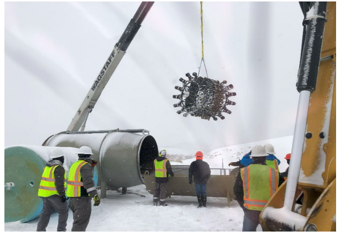
Loading the inspection into the JA-1. This tool is slowly pulled through the pipeline to measure wall thickness. It can detect anomalies as small as .25 square inches
