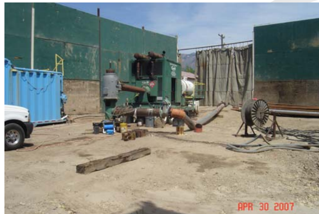
Pump test development 4500 gpm
