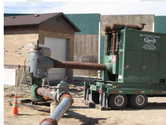
Pump Testing 3000 gpm
