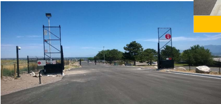
3200 West Automatic Gate
