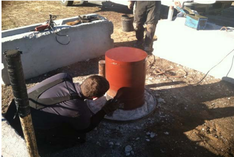
Cottonwood Street Well cap
