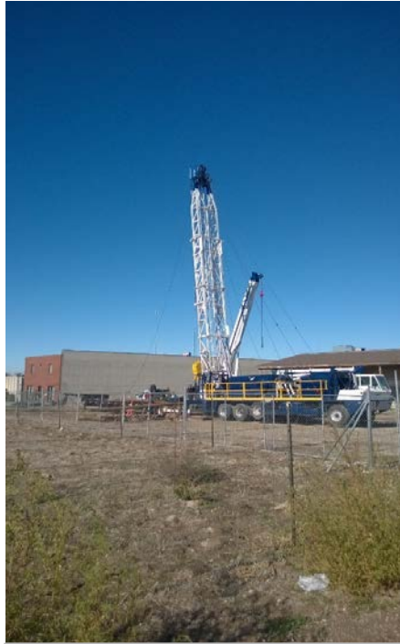
Cottonwood Street Well pump testing equipment
