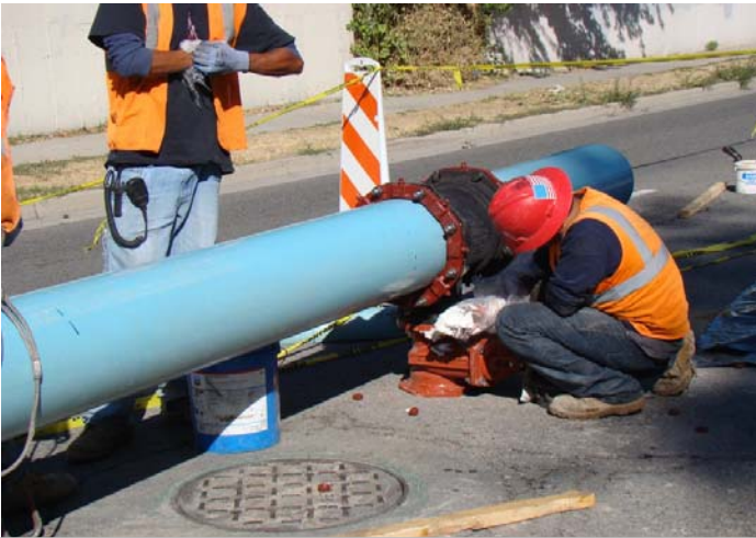
Installation of a Tee and 8-inch gate valve to tie to a mainline connection.
