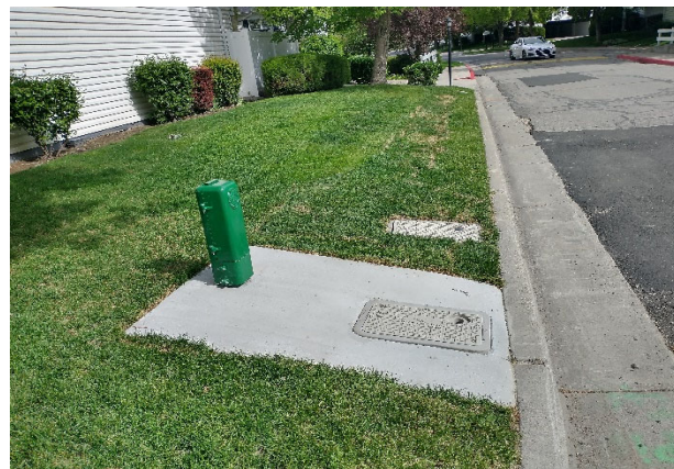
New sampling station, meter box, and turf at Old Farm
