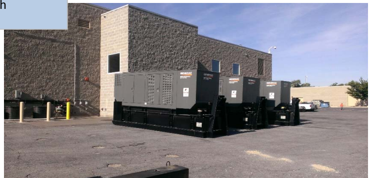
Generators parked at Vehicle Maintenance Building
