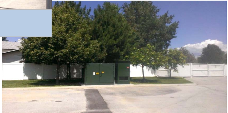
1850 East Newbury Drive Generator interface panel
